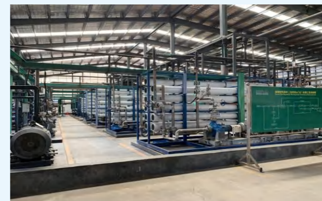
Reverse Osmosis Membrane Systems
