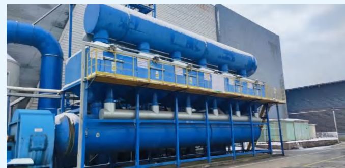
Waste Gas Treatment Facility of Jiangxi GER Co., Ltd.
