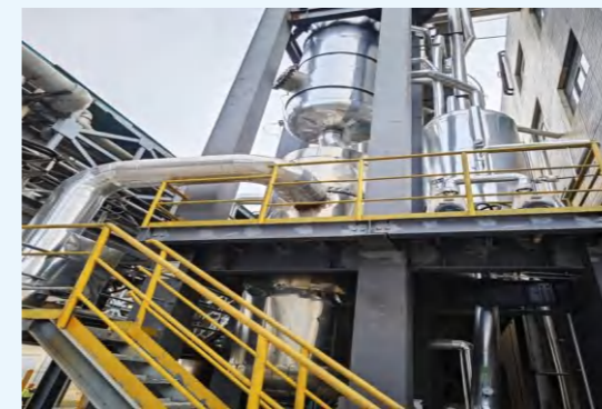
Steam stripping heat pump distillation equipment
